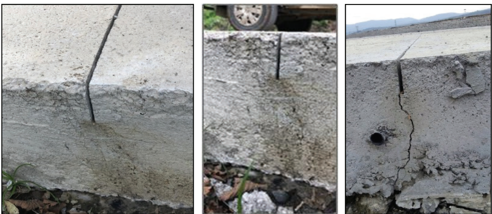
Figure 1 - Crack observation under the contraction joint in-service pavement (Trabzon/Turkey).
