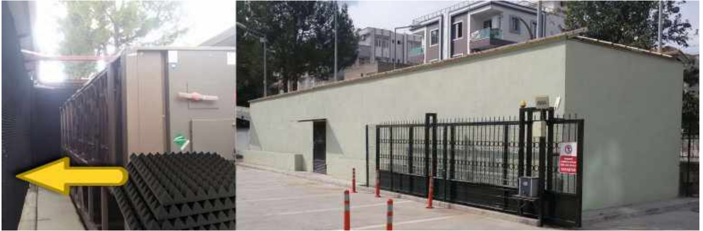
Figure 2. Isolation room for air-cooled liquid chiller noise
