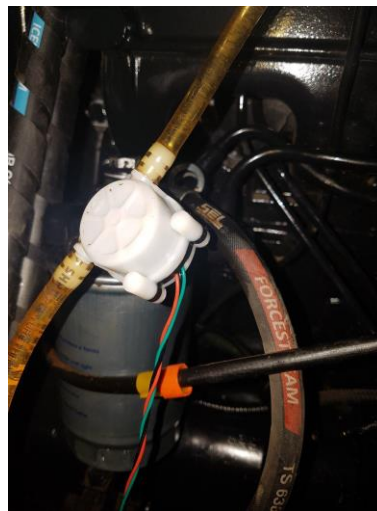
Figure 2. Flowmeter mounted on fuel line
