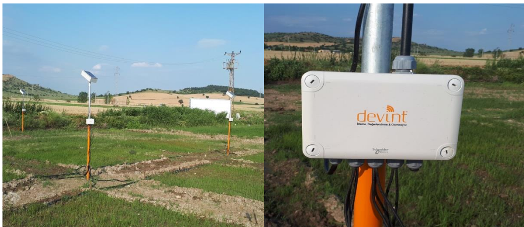
Figure 4. Remote monitoring system (DEVINT)
