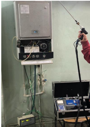
Figure 5. Analyzing gas emissions in combi boiler by ECOM J2KN analyzer
