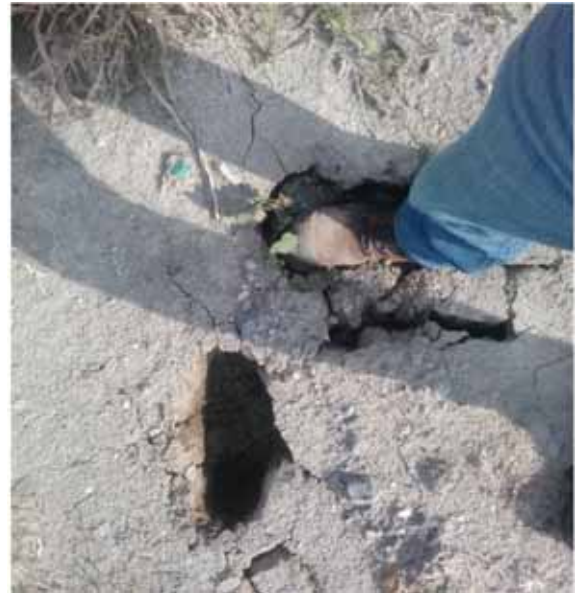
Figure 7. A photograph showing the very low soil bearing capacity of area-2
