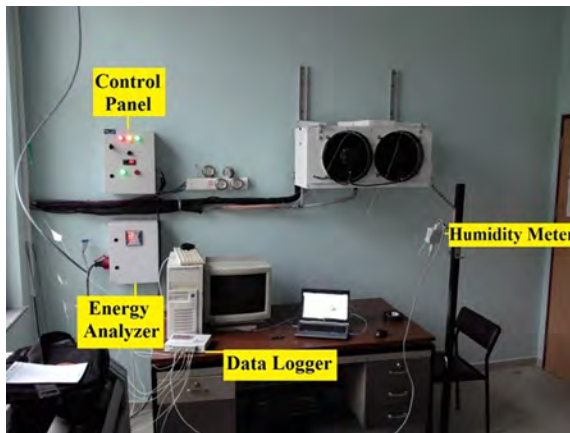
Figure 2. Indoor unit of the heat pump
