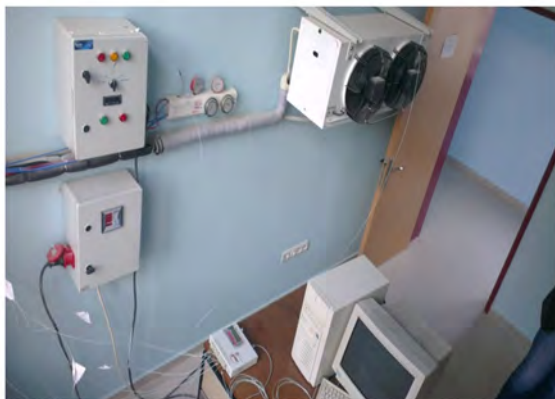
Figure 1. Indoor unit of the ASHP
