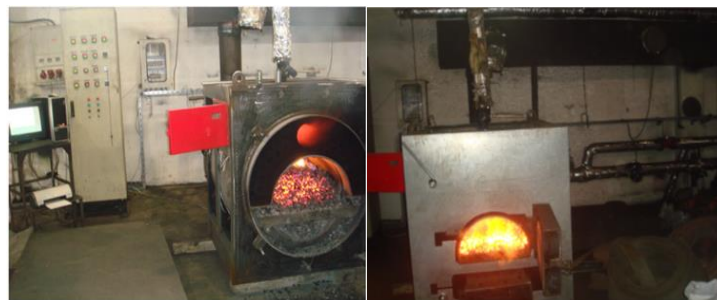
Figure 2. The boiler and automation system used in the experiments
