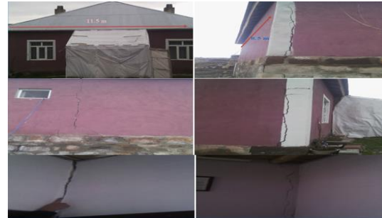
Figure 5. Damages on masonry building-3 ( 3. Yiğma binadaki hasar durumu )
