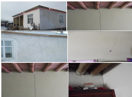
Figure 4. Damages on masonry building-2 ( 2. Yiğma binadaki hasar durumu )
