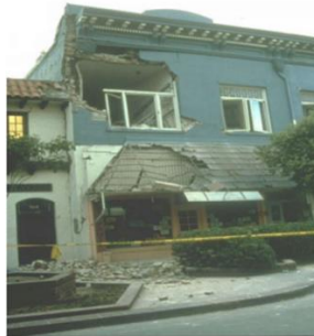
b) damage at infill walls [20]
