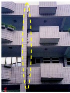
a) damage at contact [20]
