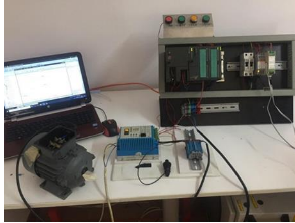
Figure 2. S7-300 PLC system connected in a laboratory environment
