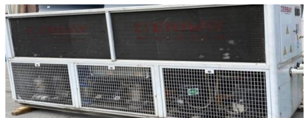
Fig. 5 Cooling system with two-compressor
