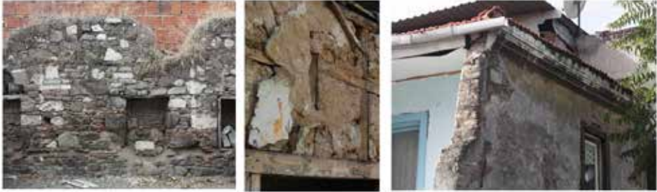
F. 11: Wall details: “d, interior facade”, “g, courtyard facade” and “f, northwestern corner” (M. Hamamcıoğlu Turan, 2015)
