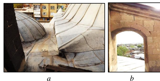
Figure 16. Openings between lead plates and segregation damages in buttresses (2021)
