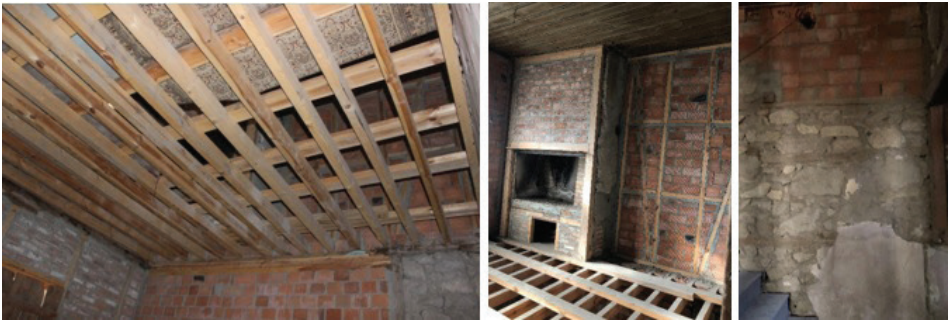
Fig. 21: Ceiling beams in site Z07 and renovated wall and floor beams and the original mud brick wall at the edge of the stairs in site 104. (By Karakuş, 2020)
