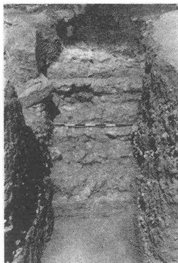
Fig. 24 Packing for podium steps on east facade of Corinthian temple. Looking west.
