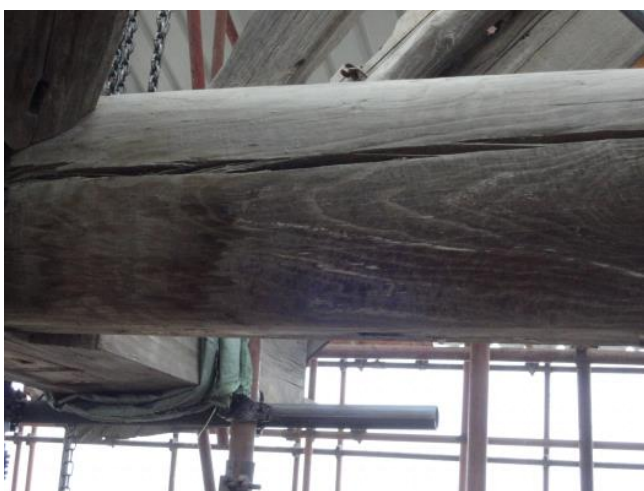
Figure 2. Cracks in square beam
