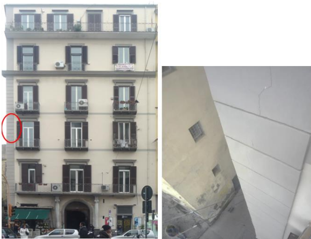
Figure 21. Crack on the corner of the main façade
