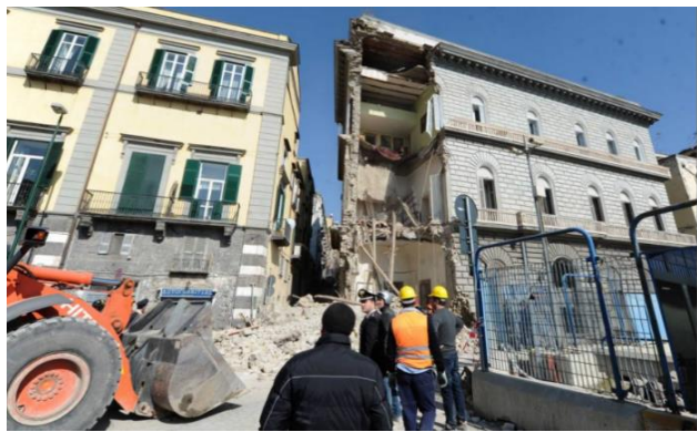
Figure 10. Neighboring building partially collapsed in 2013. Next to it is the construction site of the metro station
