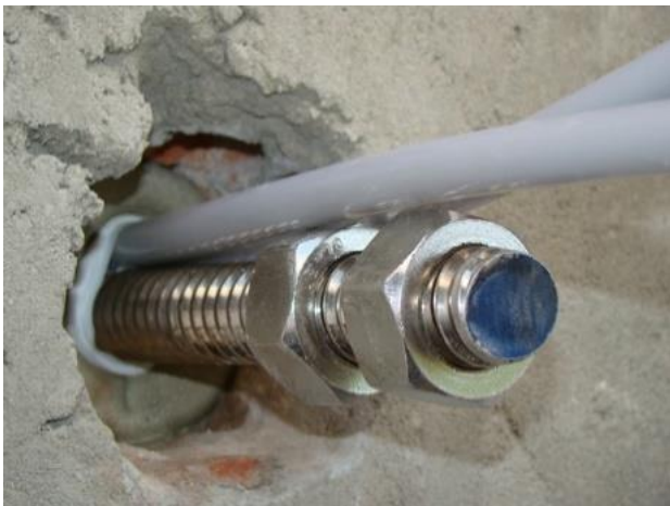
Figure 43. Anchorage in the masonry with the injection of grout limited by a sock.
