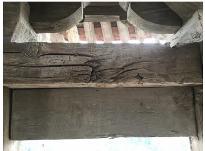
Figure 3. Damaged beam with knots
