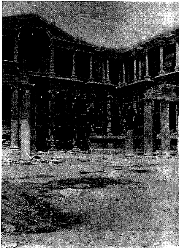
Fig. 15. Center and Northwest Corner of the Marble Court during Restoration of Pilasters, July 1971.
