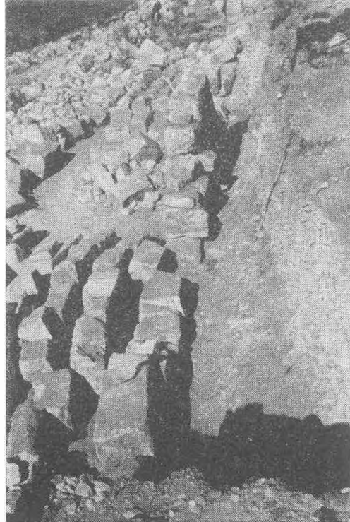
Pl. 6 — Collapsed Blocks of the Walkway Sustension Wall. To the right, the Original Sustension Wall.
