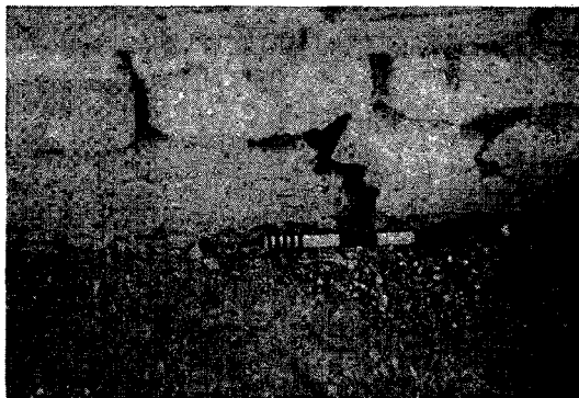
Fig. 69 — Wall of Byzantine structure to the north east of the podium displaying a crack in the wall, southwest to northeast.
