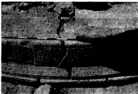
Fig. 68 — Northeast section of podium showing crack
