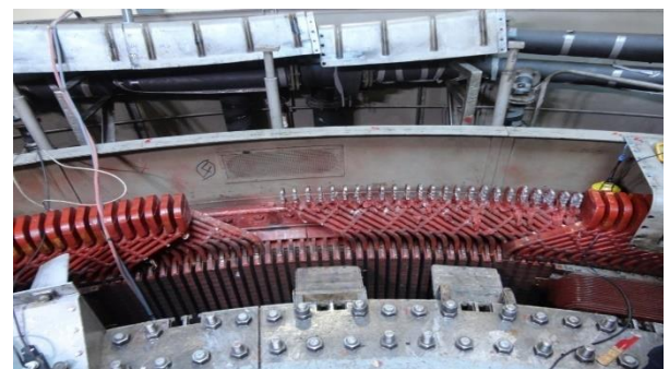
Figure 5. Generator stator windings
