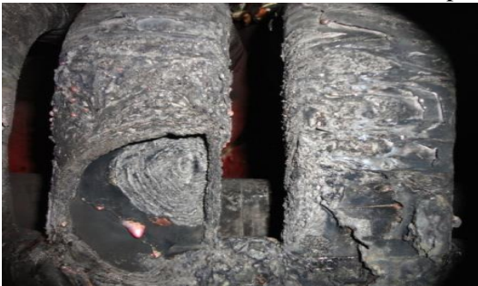
Figure 6. Fault in generator stator windings due to insulation weakening
