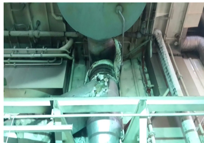
Figure 5. The funnel loop some parts of which fell off and uncovered for repairs
