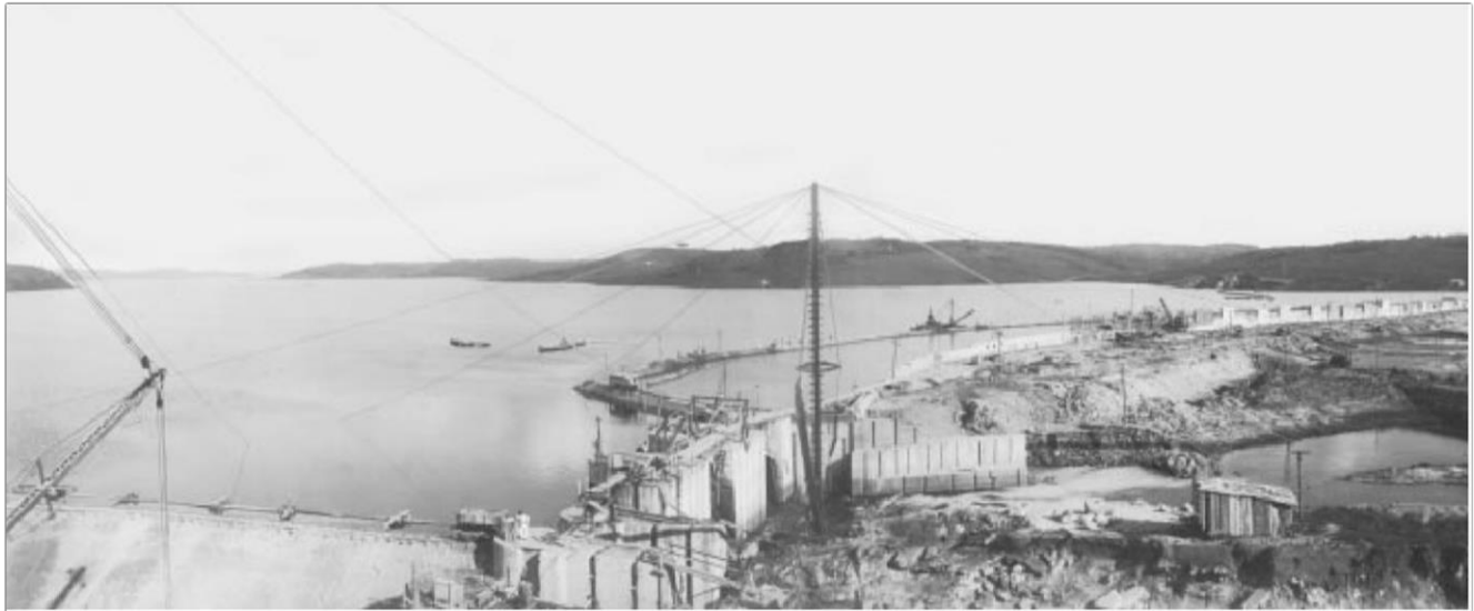
Figure 1 – Construction of Pedreira Dam at the Rio Grande water course in 1928. Source: Capobianco & Whately (2002).
