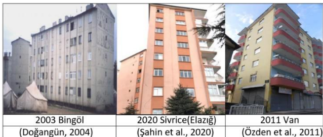
Figure 3. Negligible to slight damage for different earthquakes (Grade 1)
