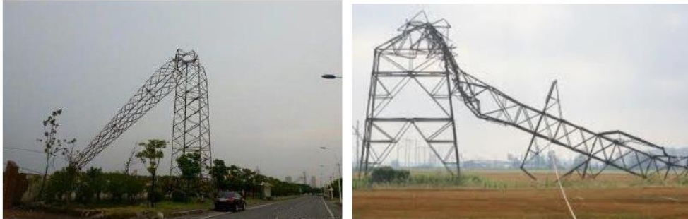
Figure 1. The steel tower damaged by the strong wind in China [1].
