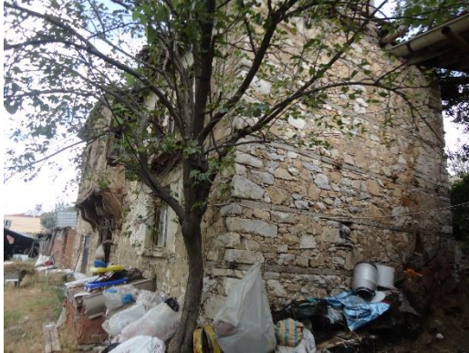
Figure 5. A typical example of a continuous stone masonry wall on the ground floor and upper floor with embedded wooden beams.
