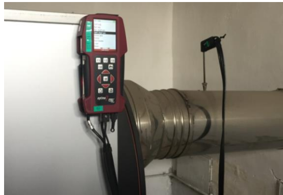
Figure 3. Flue gas analysis probe connection point.
