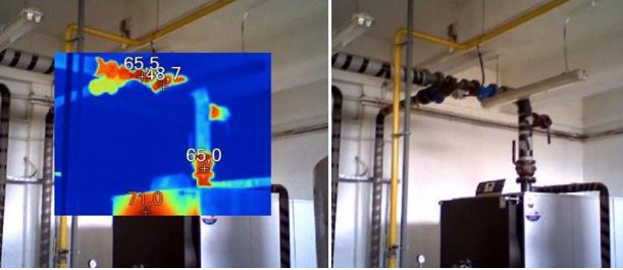
Figure 11. Thermal images of uninsulated valves.
