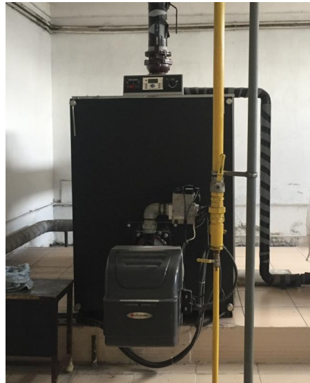
Figure 2. Existing hot water boiler.
