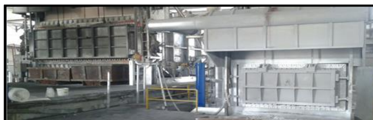
Figure 1. Melting and resting furnaces
