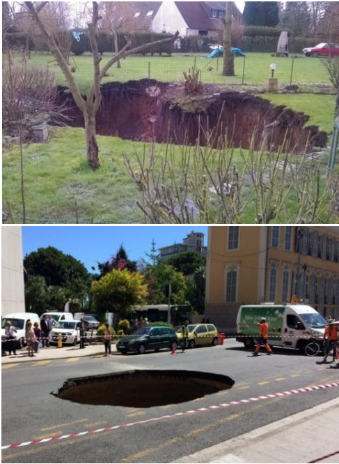
Figure. 1. Underground cavities in residential areas [9]
