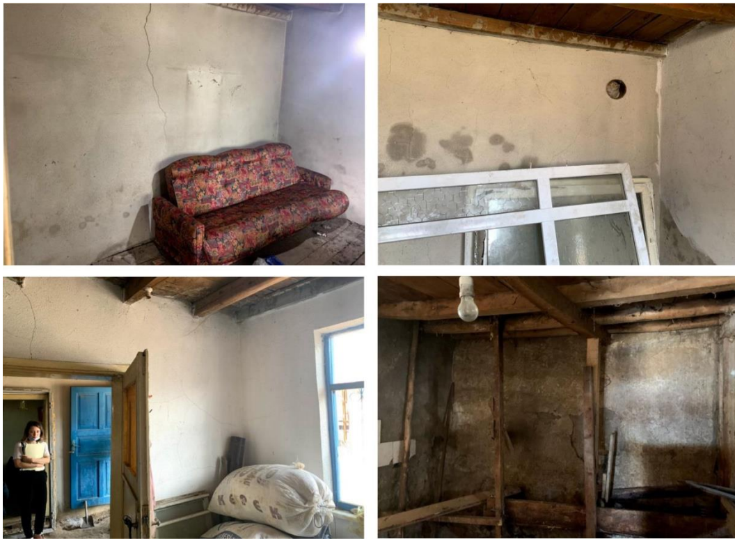
Figure 8. Damaged parts detected in the 1st building
