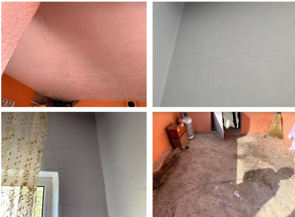
Figure 9. Damaged parts of the 2nd building
