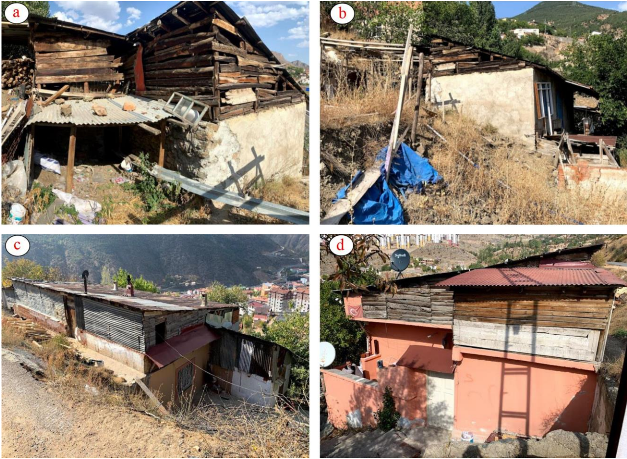
Figure 6. General views of the buildings; (a, b) 1st and (c, d) 2nd building
