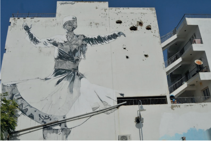
Photograph 8: This building was damaged during war times, bullet and bomb marks can be easily seen. However, the artist of this mural drew this image of a whirling dervish intentionally not wanting to cover the marks since, as explained in an interview, peace and war wanted to be emphasized together.
