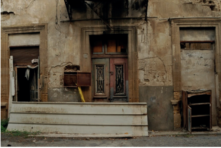
Photograph 3. An abandoned house in Nicosia Walled City.
