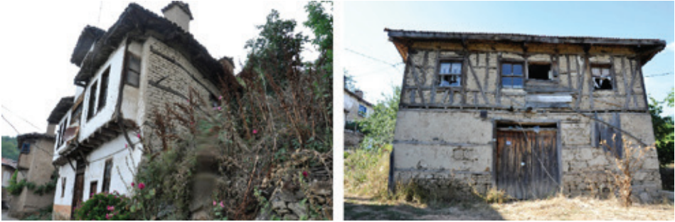
F. 7: Examples of traditional structures built with stone, soil and wood in Dağgüney and Süleymanbey villages (Güneş Kaya, 2019)
