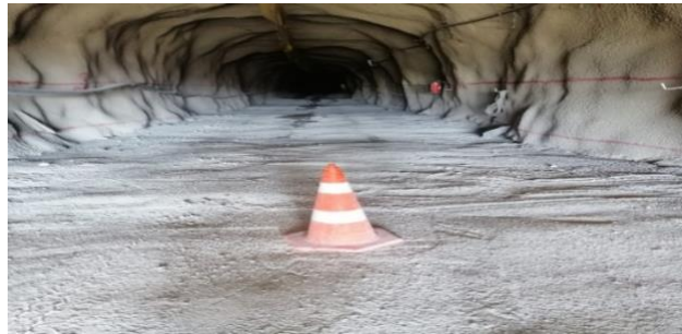
Figure 4. Conical object used in the transformation of the point cloud obtained from laser scanning.
