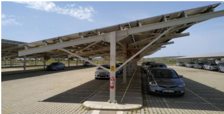
Figure 3. Angle of PV panels with ground.
