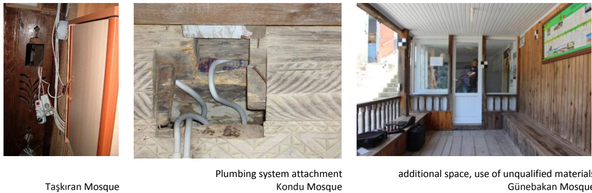
Figure 6. Examples of human-induced deformation of wooden materials in wooden mosques
