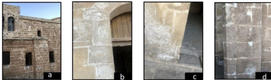
Figure 4. Physical deterioration of Hatuniye Madrasah (Biçen Çelik, 2019)
