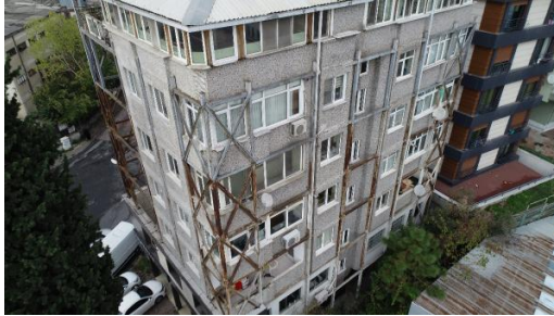
Figure 4. Seismic Bracing Example applied on a residential building at Istanbul, Turkiye (URL-4).
