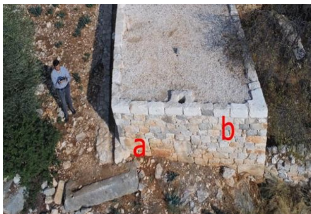
Figure 5. Change of color on the west facade (a), surface contamination (b)
