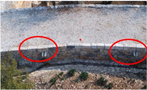
Figure 8. Surface loss in gutters in the structure
