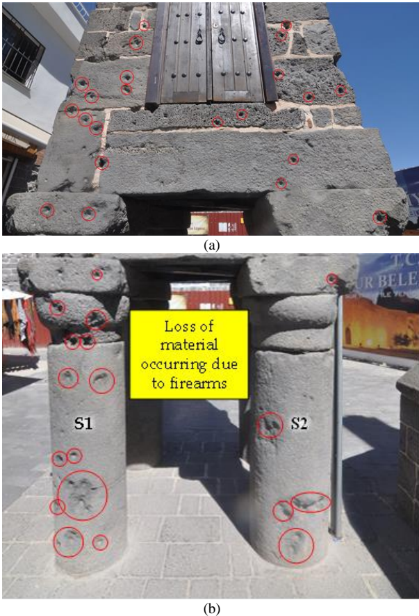
Figure 10. Photographic views of damages caused by firearms on: (a) the body and (b) columns of the Four-Legged Minaret (taken in 2021)
