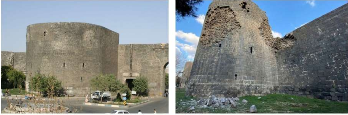
Fig. 6. a-b. Diyarbakır Castle, after the February 06, 2023 earthquake (Arkeofili, 2023).
