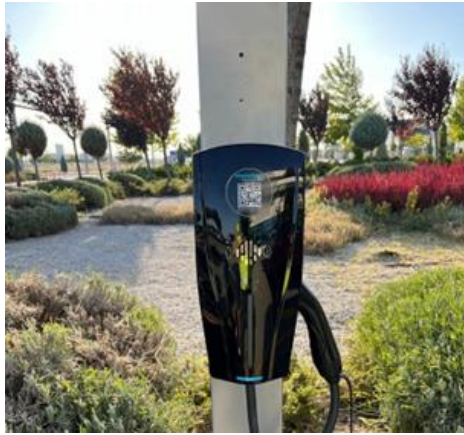
Fig. 5. Installation image of 22 kW AC type 2-socket charging station.
