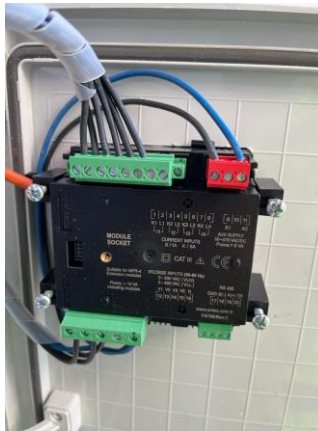
Fig. 4. Energy analyzer installation visual on the panel.
