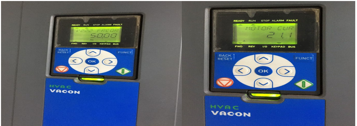
Figure 1. Electric motor frequency and current at 35.9°C ambient temperature
