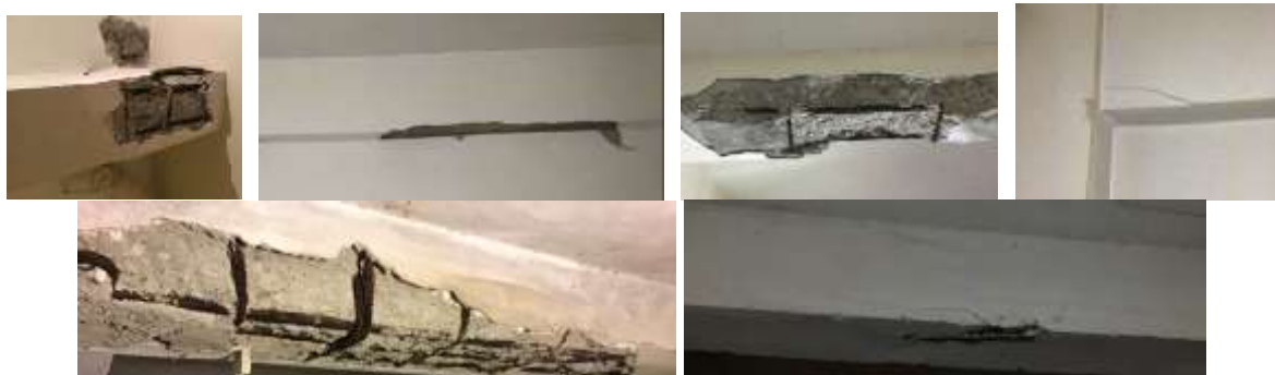
Figure 1. Images of corroded RC beams
