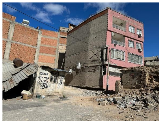
Figure 5. Damaged masonry walls in Adiyaman city center
