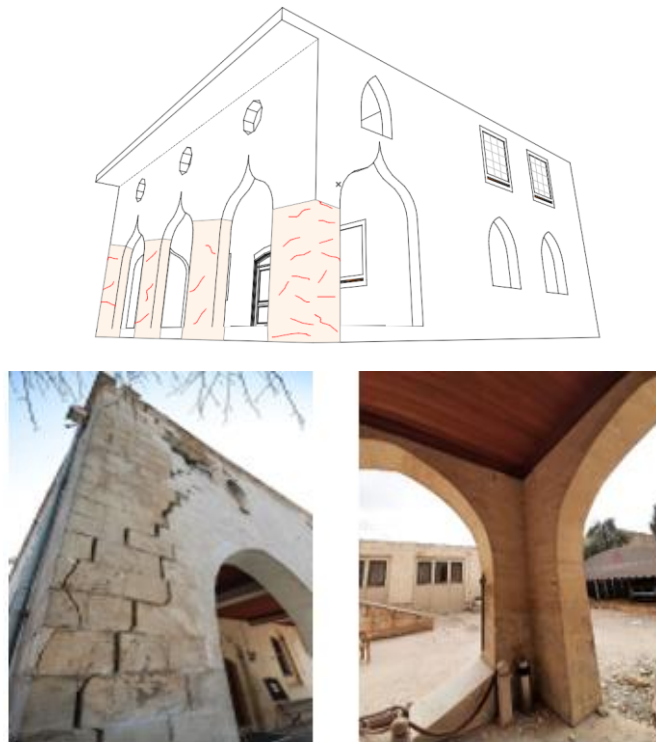
Figure 8. In the column bases, in-plane torsion or shear cracks (3b) are observed
