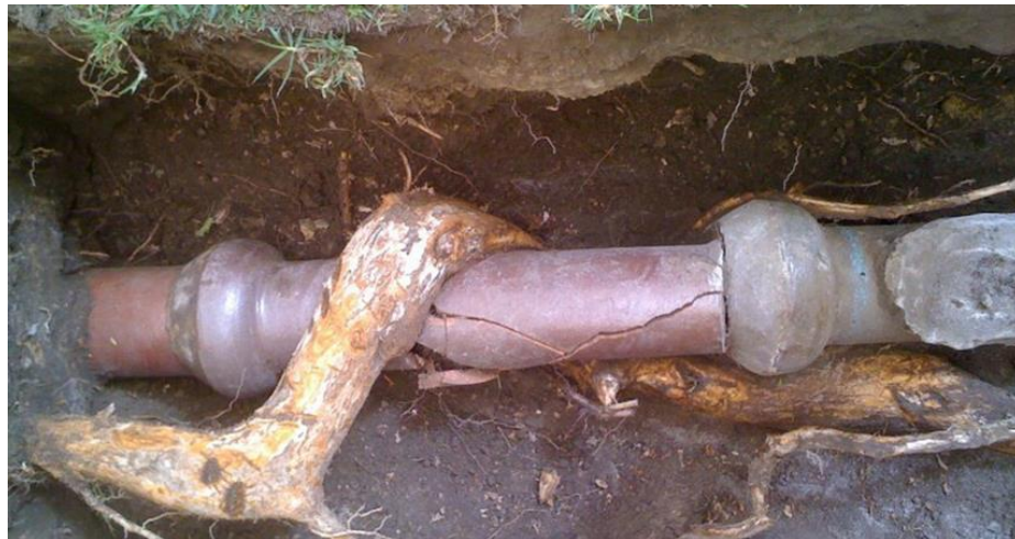
Figure 4. Effects of tree roots on sewer line (911HVAC, 2019)
