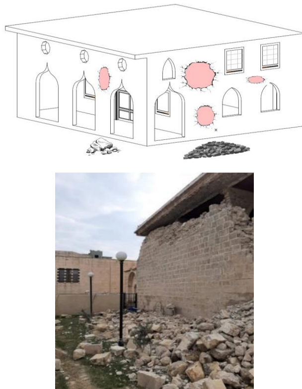
Figure 2. Fragmentation or loss of stone materials in the wall (2a)
