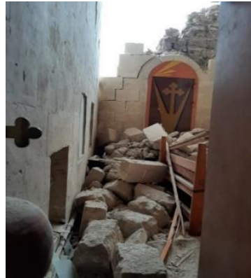
Figure 3. Weathering of the surface coating (2b), especially in double-walled stone walls
