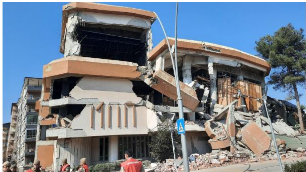
Figure 9. Hatay Cultural Center damaged after 6 February 2023 Earthquakes (TMOBB, 2023)
