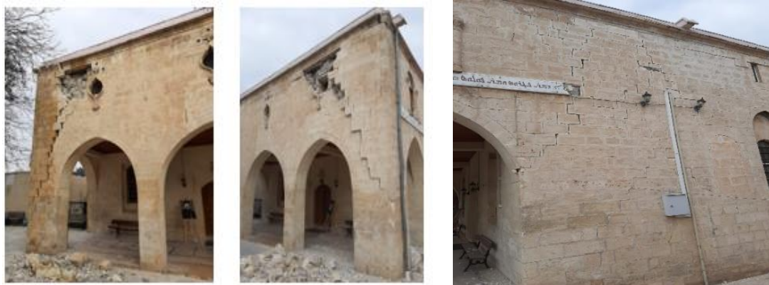
Figure 5. Shear cracks in the facade wall (2e)
