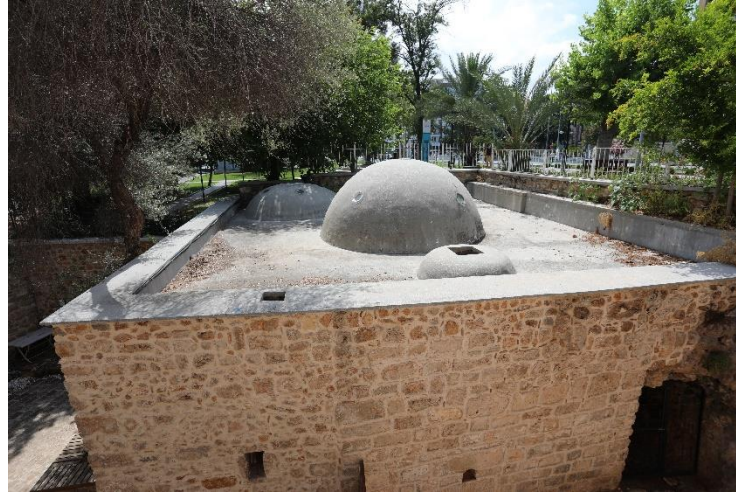
Figure 3. General view of the upper covers of the Yivli Minaret (Mevlevihane) Bath
