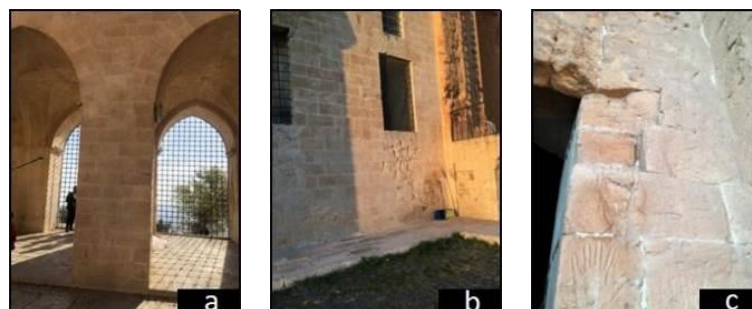
Figure 8. Anthropogenic deterioration of the Kasımiye Madrasah (Biçen Çelik, 2019)
