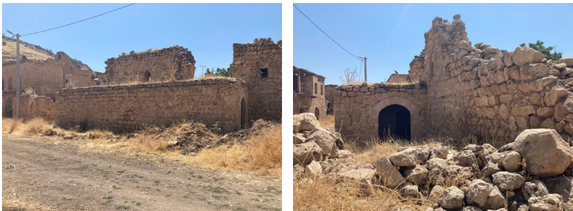
Figure 7. Deteriorations observed on parcel 1-2 of plot 179
