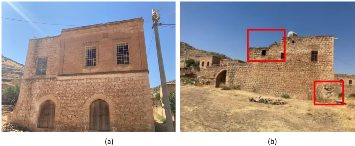
Figure 10. Deteriorations observed on the facade of parcel 1 on plot 186
