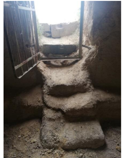
Figure 15. The Saklı Church, ladder distortion detail (Ertürk, 2020, p.145)
