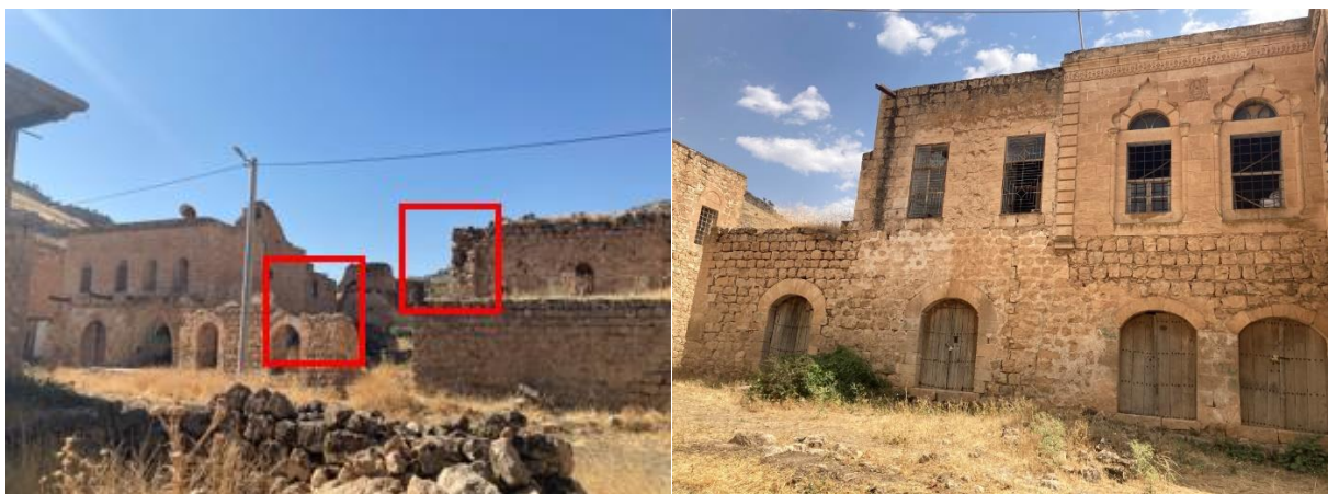
Figure 8. Deteriorations observed on parcel 3-4-5-6 of plot 179
