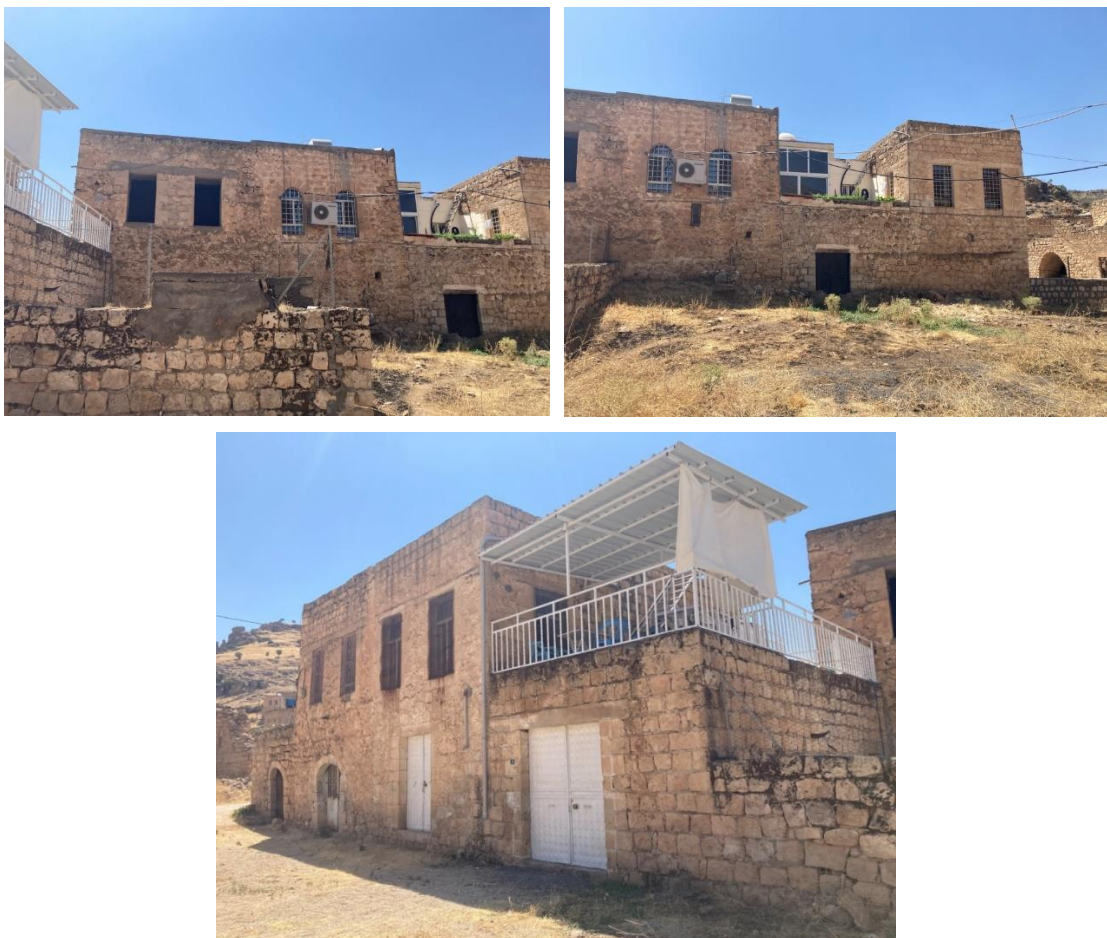
Figure 9. Deteriorations observed on parcel 3-4-5-6 of plot 179
