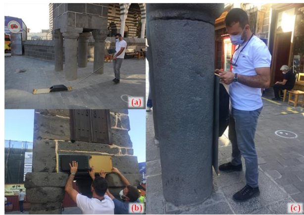
Figure 8. A typical application of the GPR on: (a) the ground of the surrounding area of the minaret, (b) the basalt lintel of the minaret, and (c) the column of the minaret
