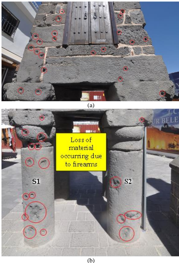
Figure 10. Photographic views of damages caused by firearms on: (a) the body and (b) columns of the Four-Legged Minaret (taken in 2021)
