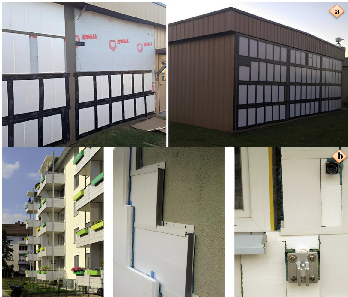
Figure 2. a) Low-cost VIPs for energy-efficient retrofit of external walls [23], and b) hybrid external wall insulation of VIPs with EPS foams [24].
