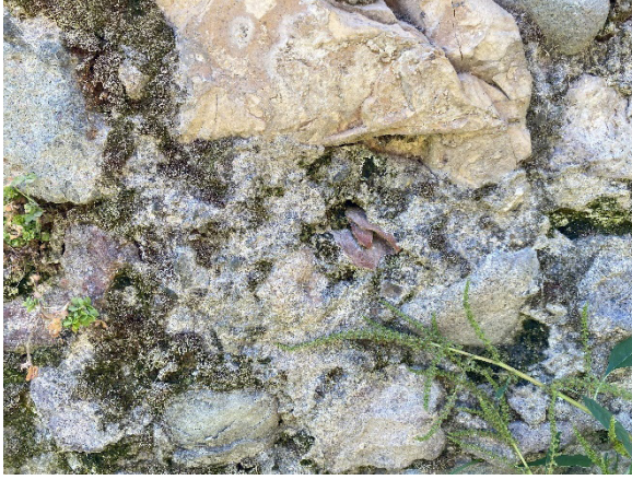
Figures 6–8. Perimeter wall that supposedly remained from the former Greek cemetery of Burhaniye, partially Sevgi Park today (Adramyetteion Researches, 2023).
