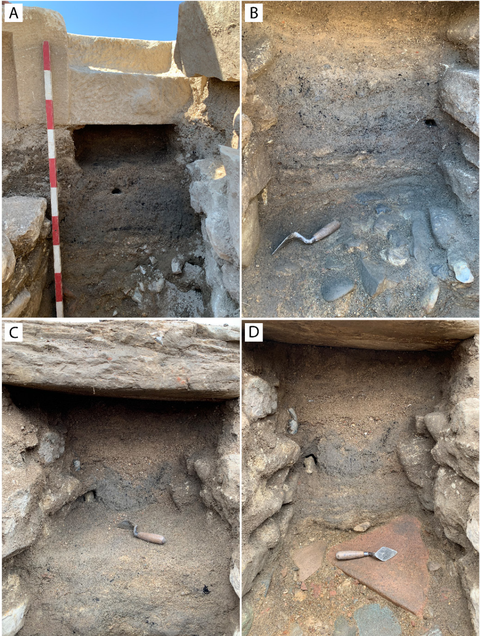
Fig. 10: Sewer upper part: a.Sewer fill; b.Stone base under the cocchiopesto floor revetment which was eroded in time due to water stream; Sewer lower part: c.Sewer fill; d.Tile base under the cocchiopesto floor revetment which was eroded in time due to water stream
